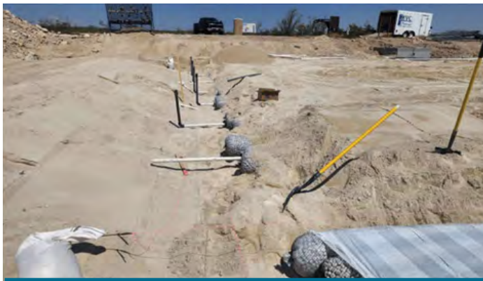
Evapotranspiration Bed end view of distribution bundles
