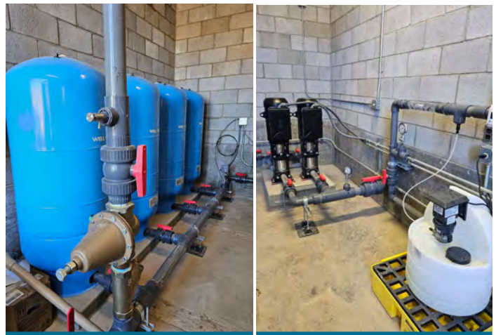
At Left: New pressure tanks
