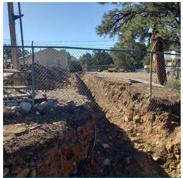
Heron Lake Water Treatment Plant in background
